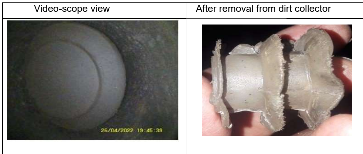
Blockage in BP pipe
