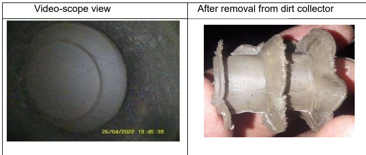
Blockage in BP pipe
