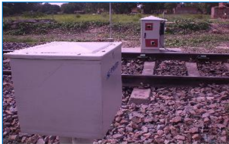
Typical Installation of Hot Box detector
