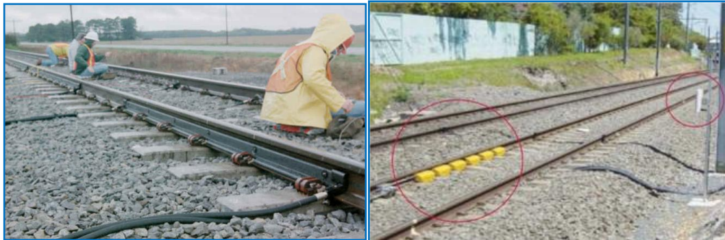
Typical installation of Wheel Impact Load detector (WILD)
