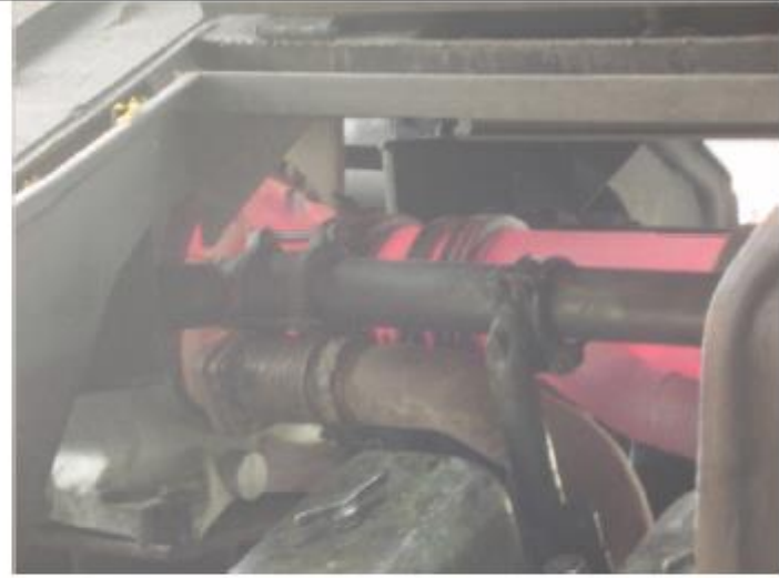
Gas inlet casing is also red-glowing → indication for extremely high temperature
