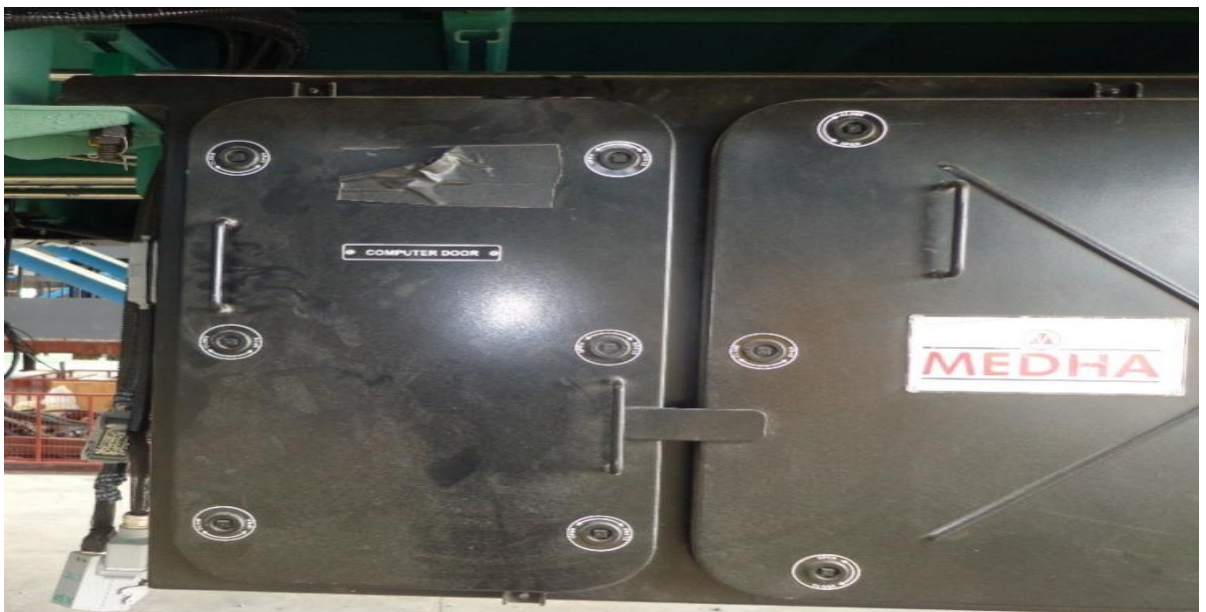
Fig6.0k: Line &amp; Traction Control Unit (LTCU)
