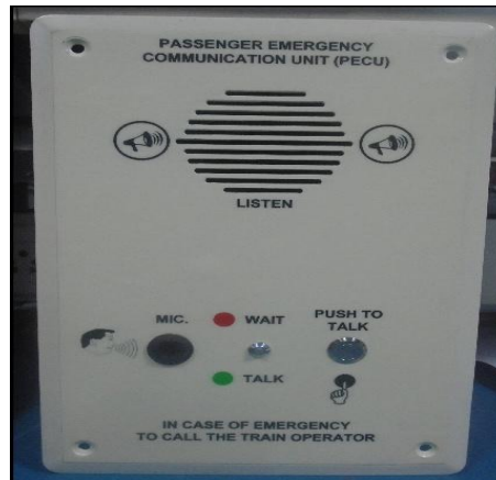
Fig7.0g: Passenger Emergency Communication Unit (PECU)
