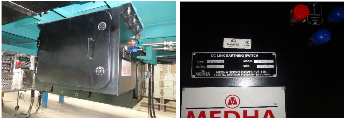
Fig6.0i: DC link earthing switch
