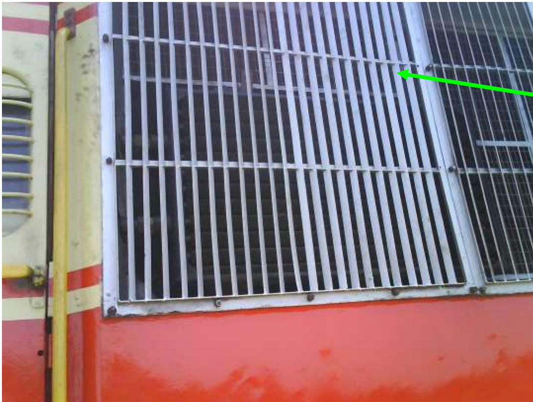
HYDRAULIC OIL COOLER
