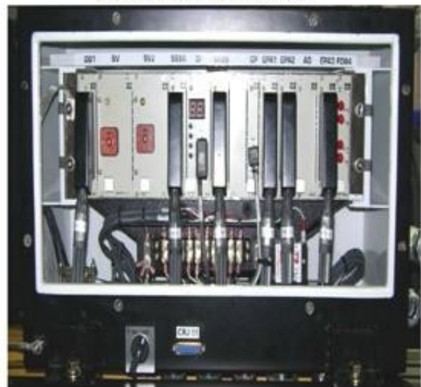
COMPUTRE RELAY UNIT
