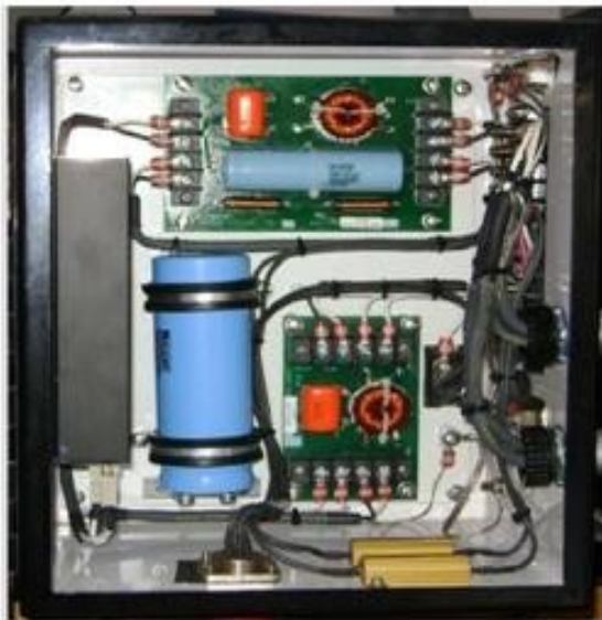
VOLTAGE CONDITIONING UNIT
