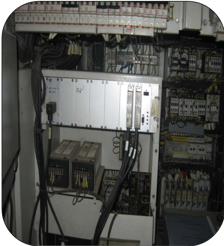
WSP control panel/Micro Processor
