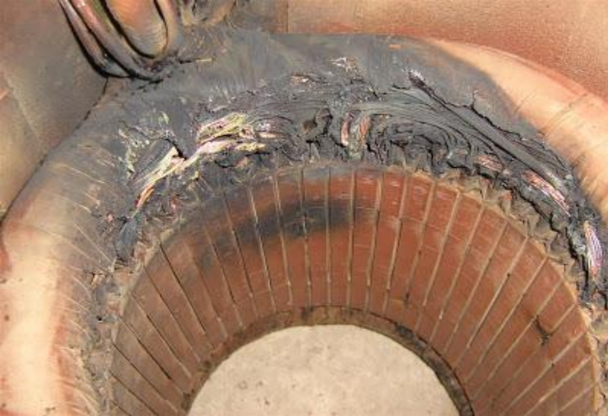
Result of Insulation Failure
