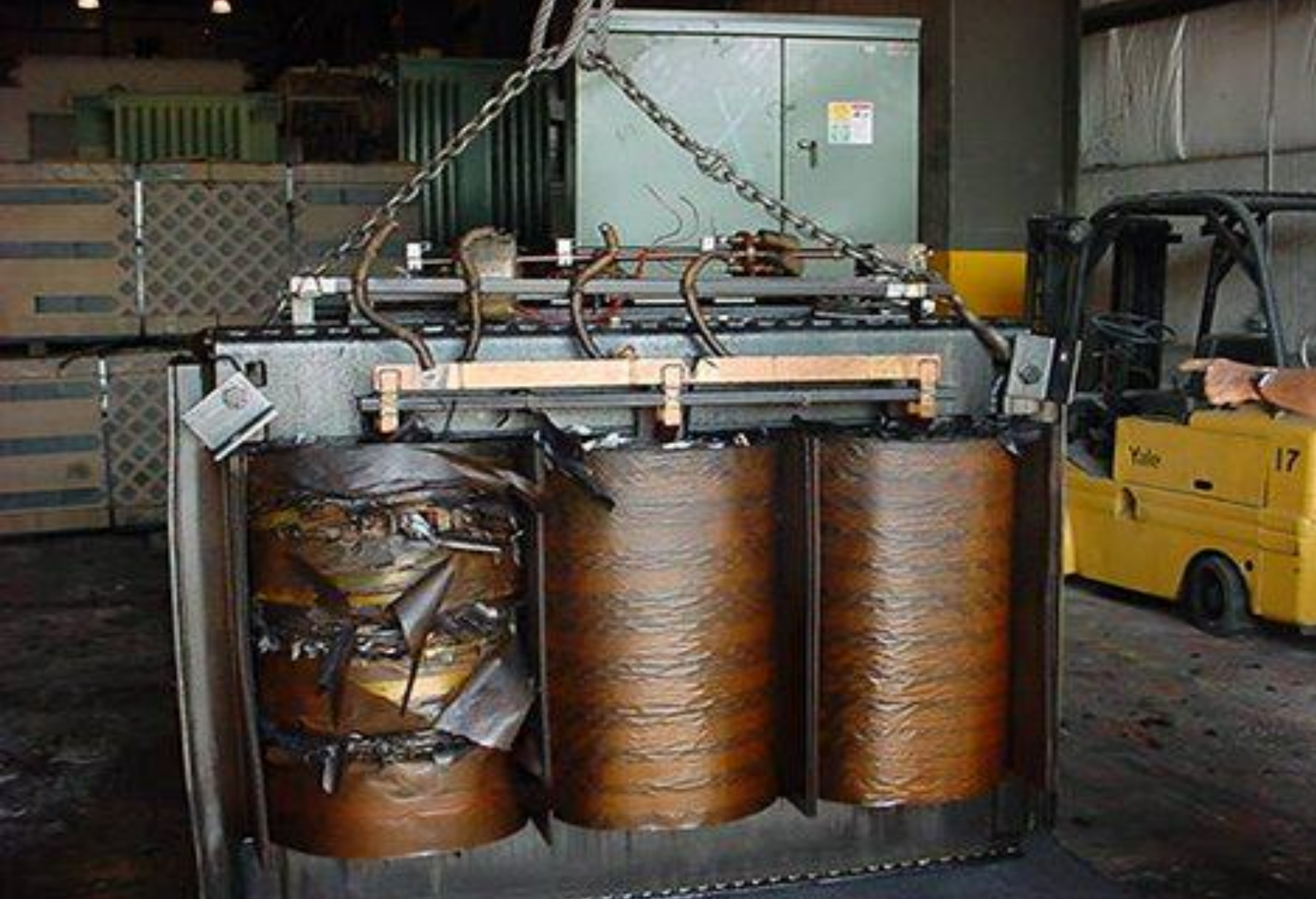
Result of Insulation Failure
