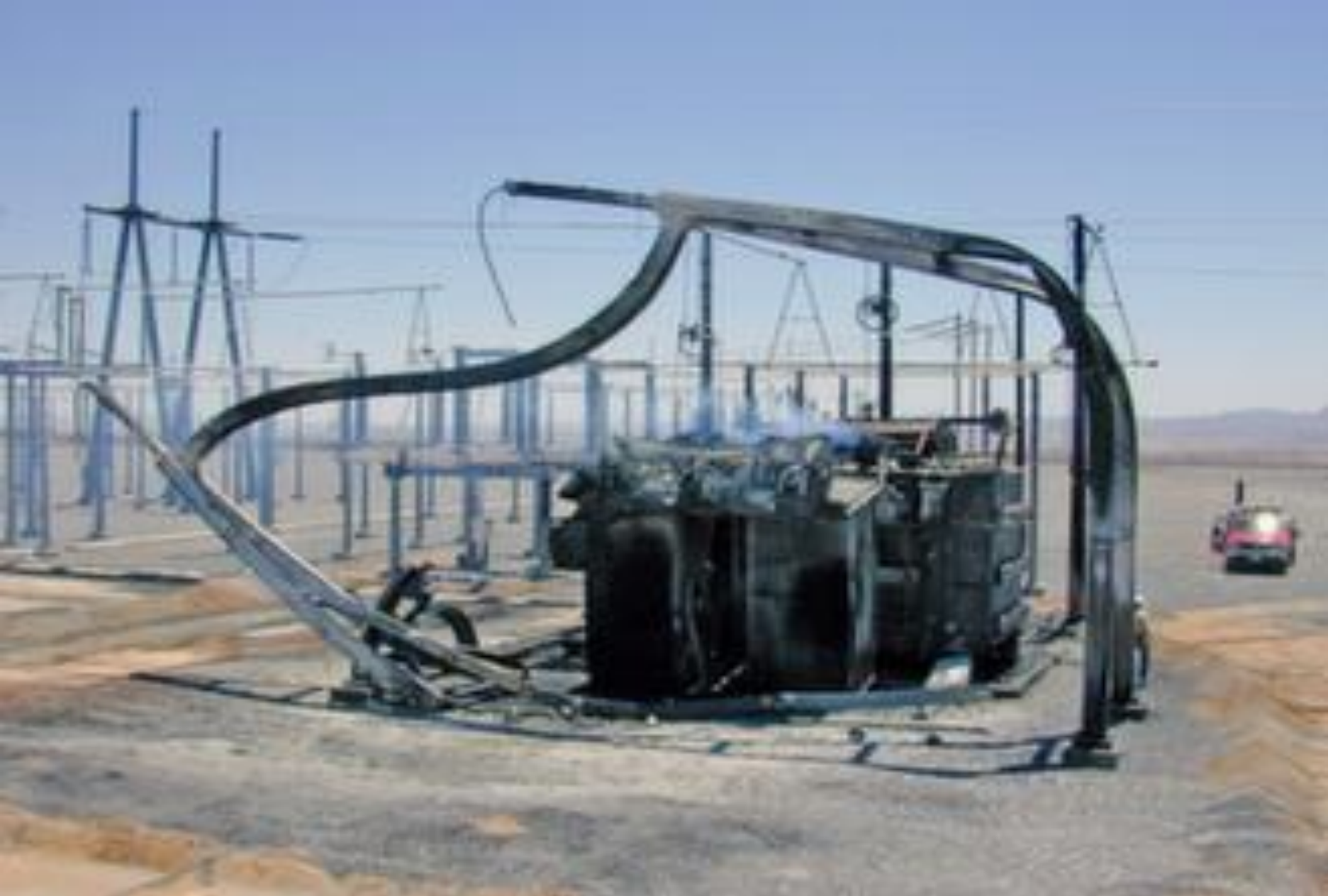
Result of Insulation Failure
