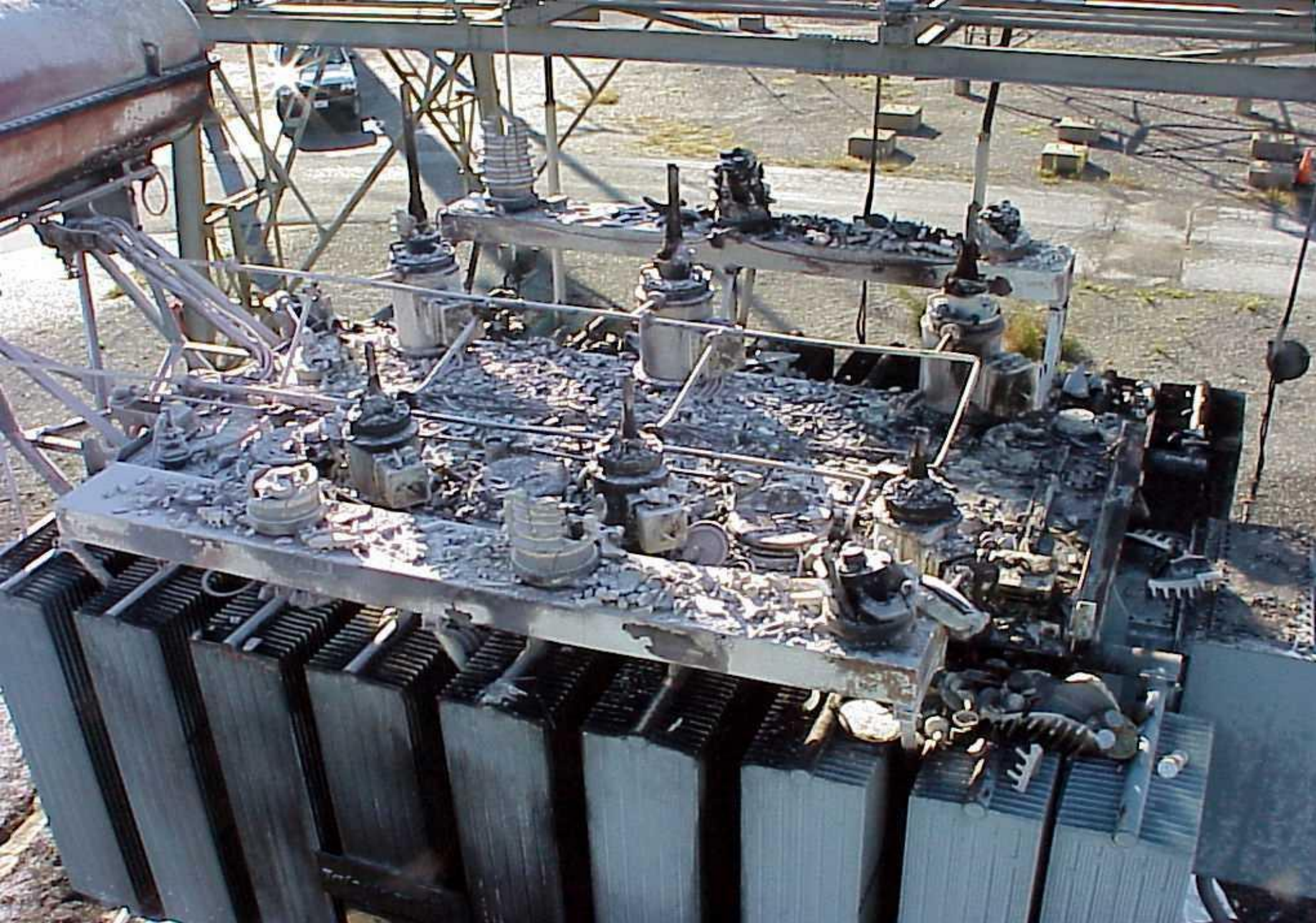
Result of Insulation Failure
