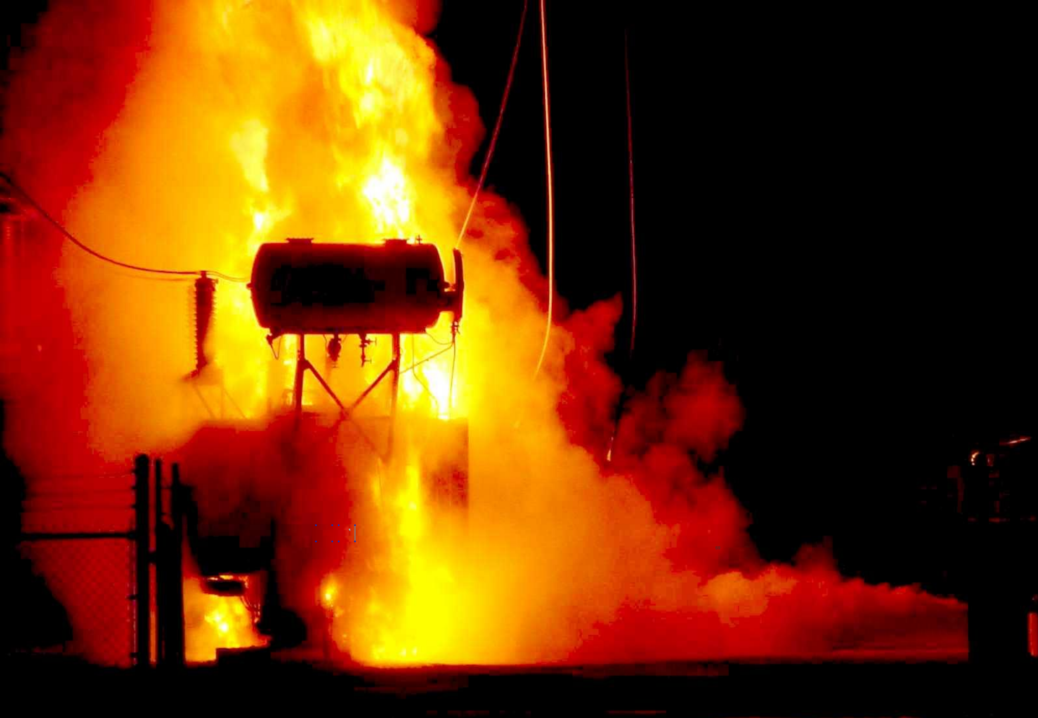
Result of Insulation Failure
