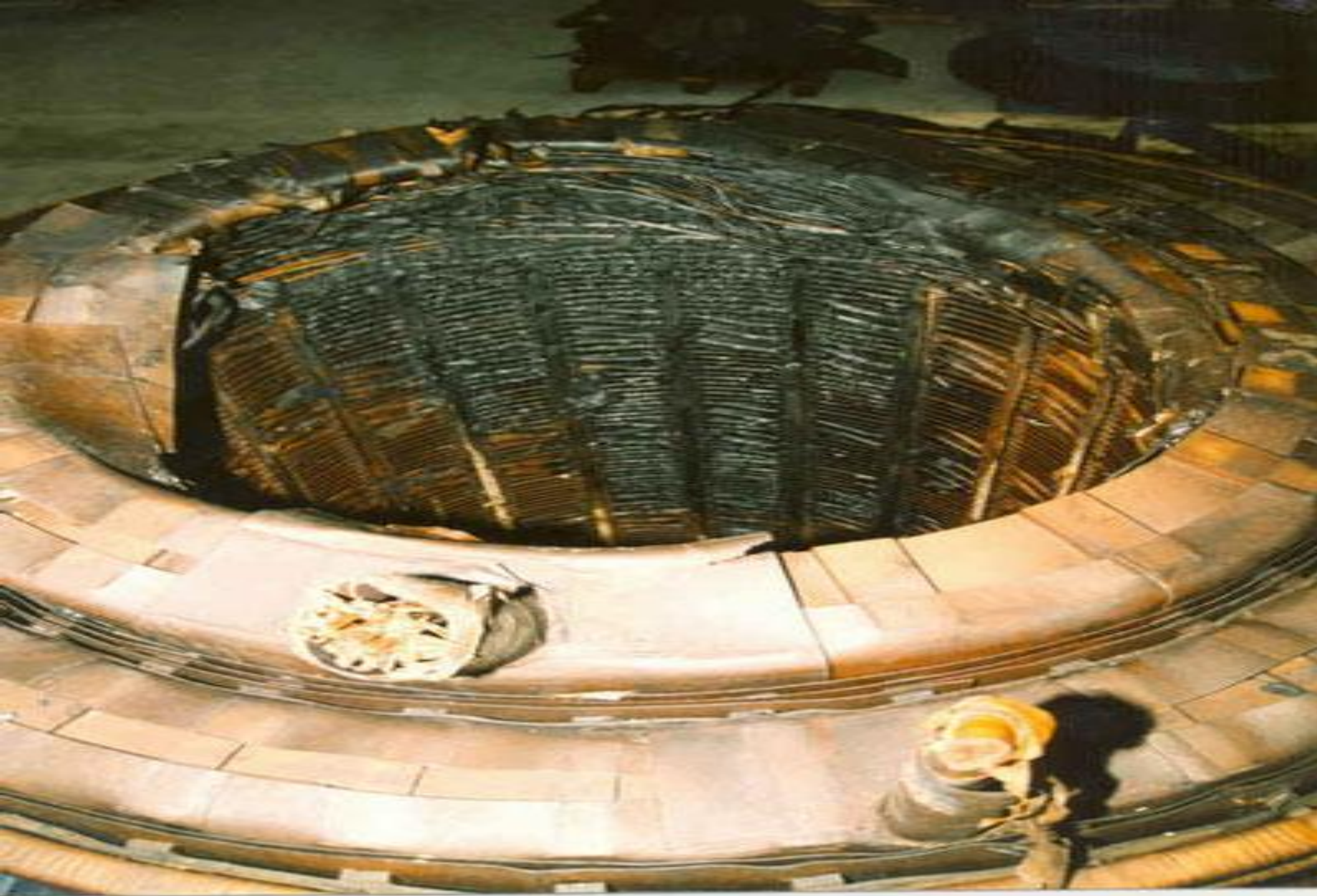
Result of Insulation Failure
