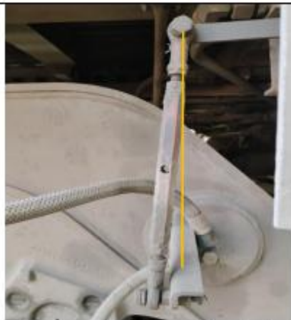
Improper Welding of Brackets
