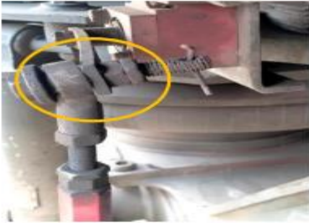
Cause no.01 -Totally tightened. No space for ball movement
