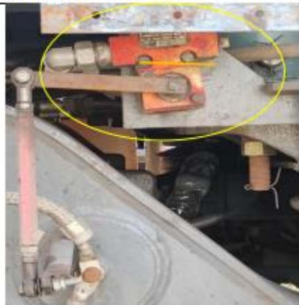
Misalignment of mounting Holes
