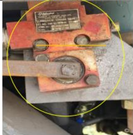
Misalignment of mounting Holes
