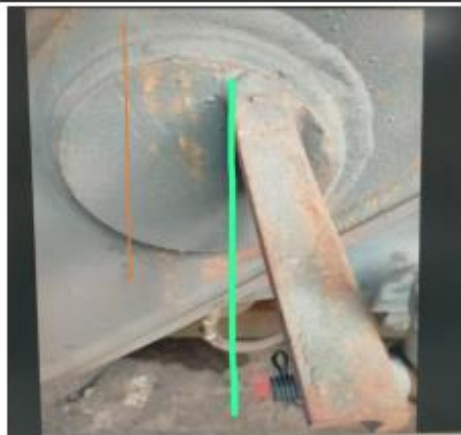
Improper Welding of Brackets
