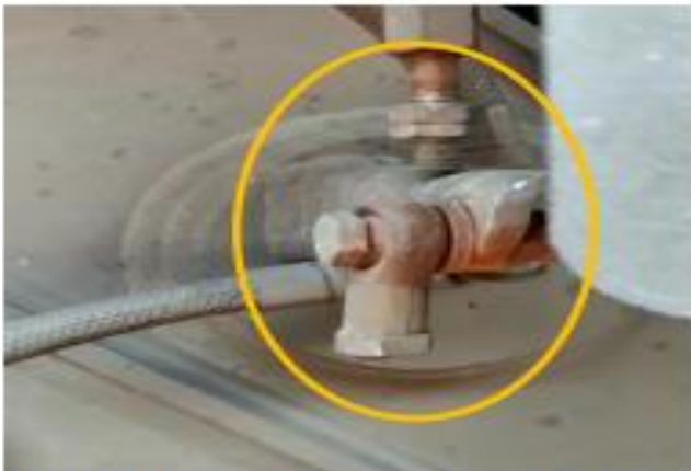
Resulting in -Installation Lever Broken
