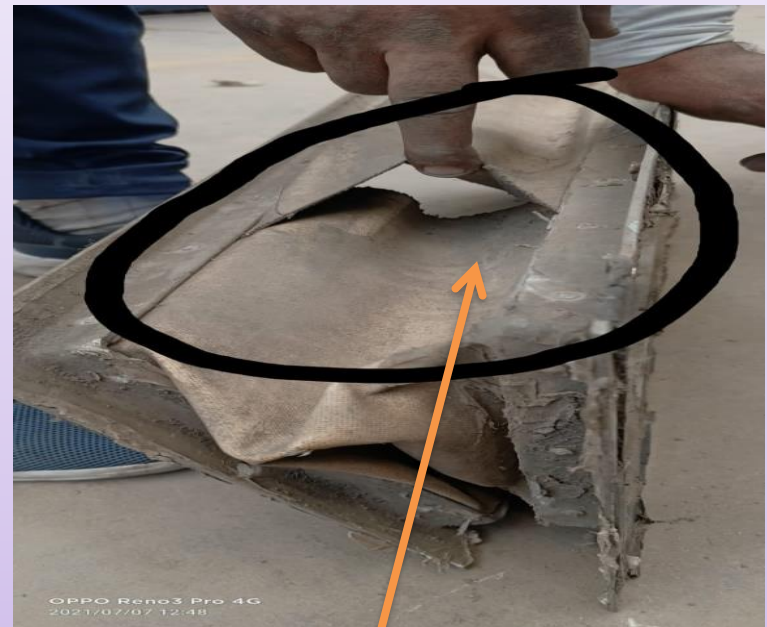
99153 NPP side Supply air
