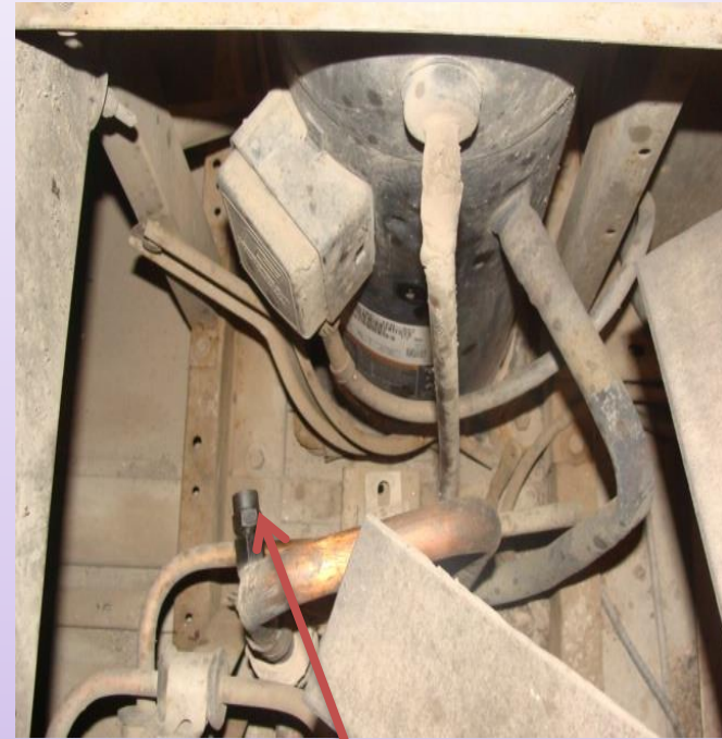
Gas charging valve
