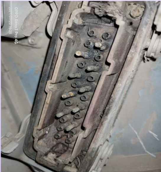
SHORT due to ingress of rain water
