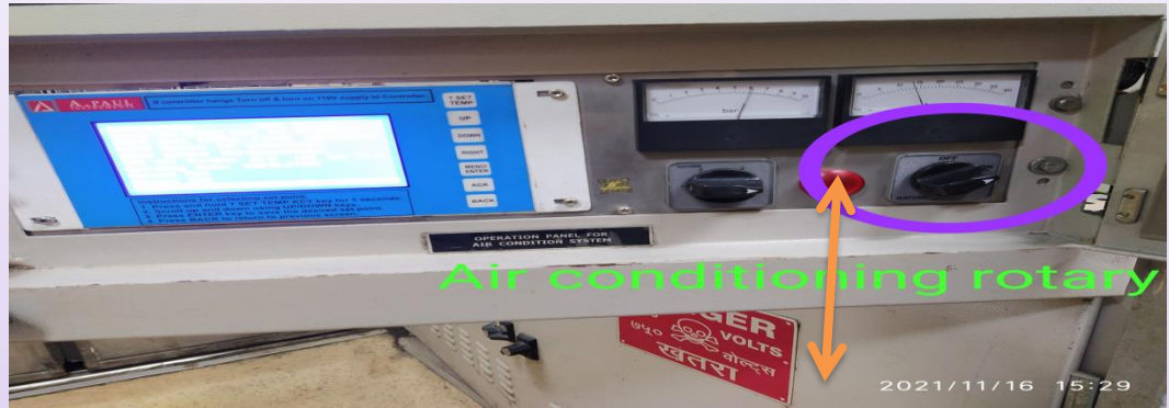
Fault indication lamp
