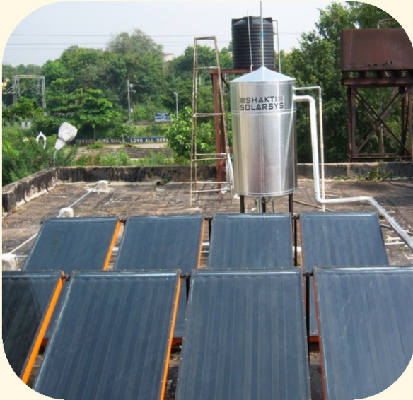
Solar Water Heater For Canteen
