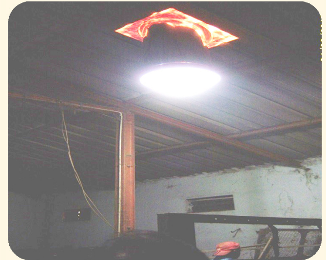
8 nos Natural Light Pipes in Stores Ward No.09 & 02
