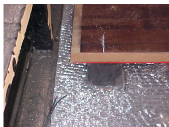
Flooring boards resting on Rubber De- Coupling elements
