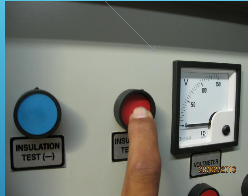
DC Positive side Insulation
