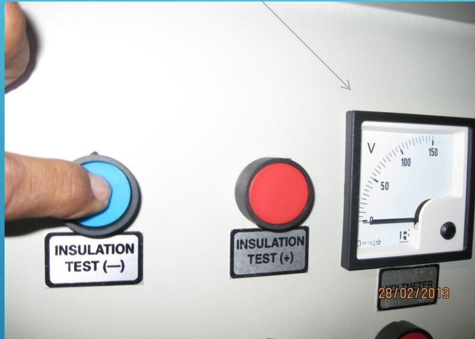
DC Negative side Insulation
