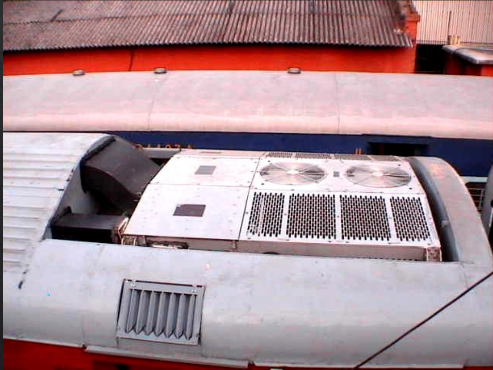
Fresh air intake grill
