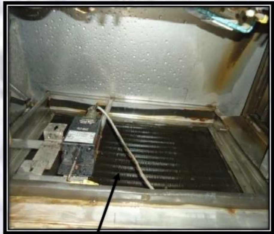
Evaporator coil after cleaning
