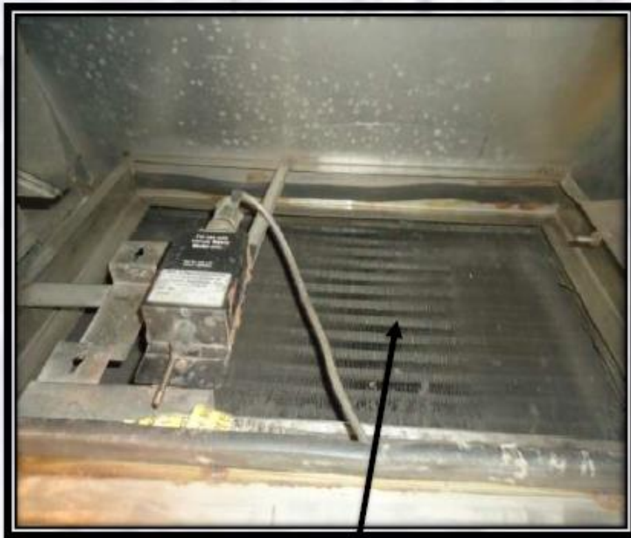
Evaporator coil before cleaning
