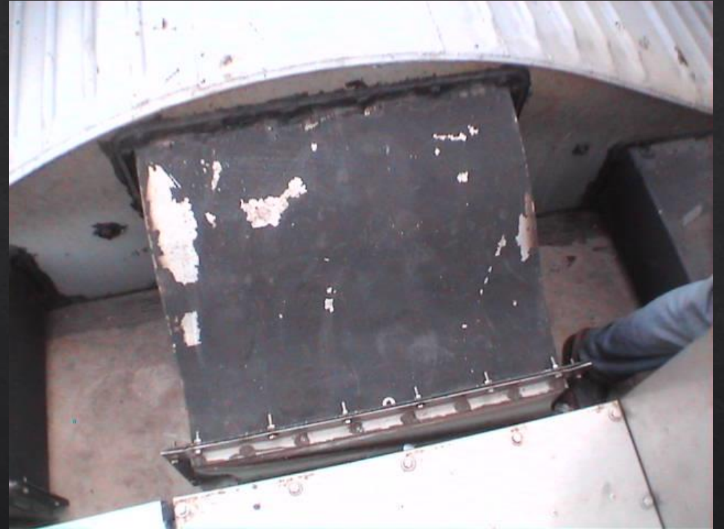
Supply air duct
