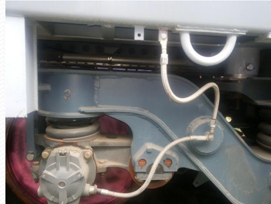
Shell body to bogie frame earthing cable
