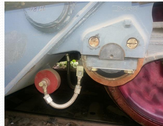
Resistor earthing cable
