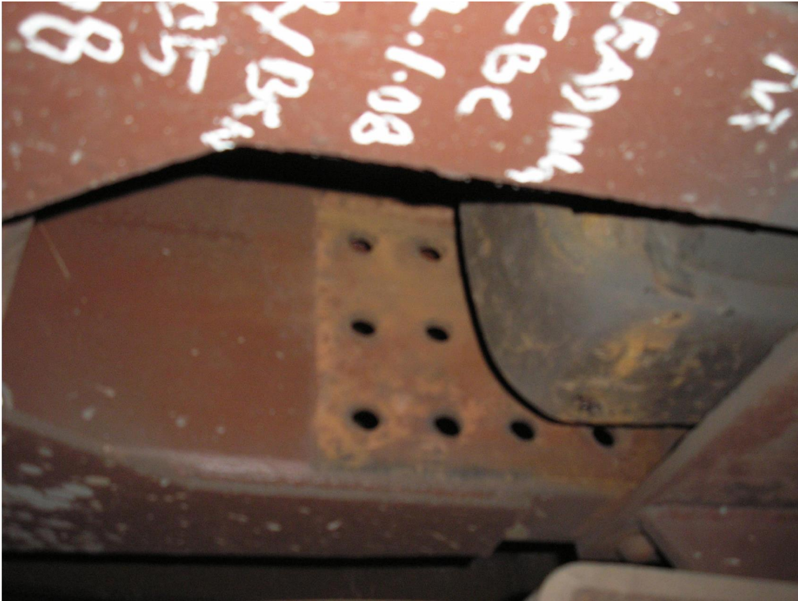
RIVETS SHEARED - OFF & REAR STOPPER MISSING
