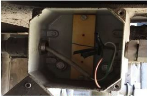
Missing WAGO Terminal
