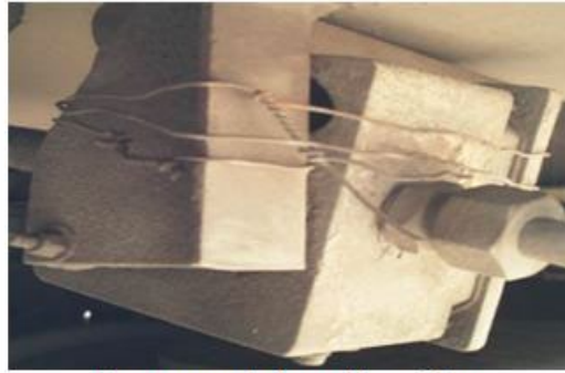
Damaged Junction Box
