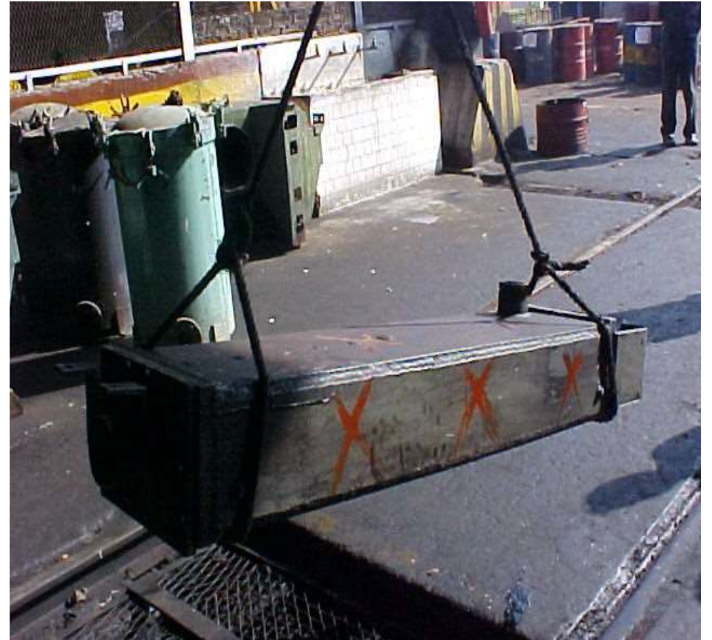
Corroded Lube oil Cooler
