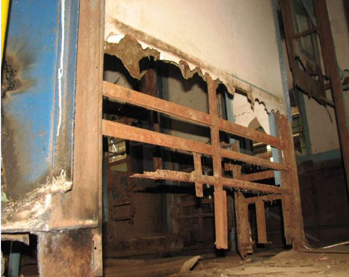
Corroded Lavatory Wall
