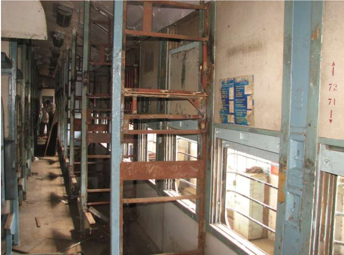
Corroded Body Pillar Structure
