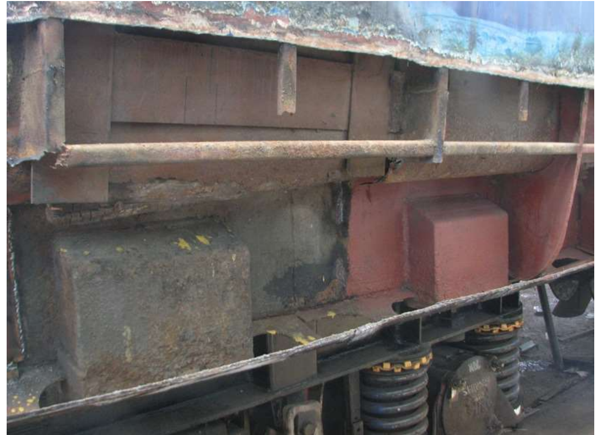
Corroded Side Wall & Turn Under
