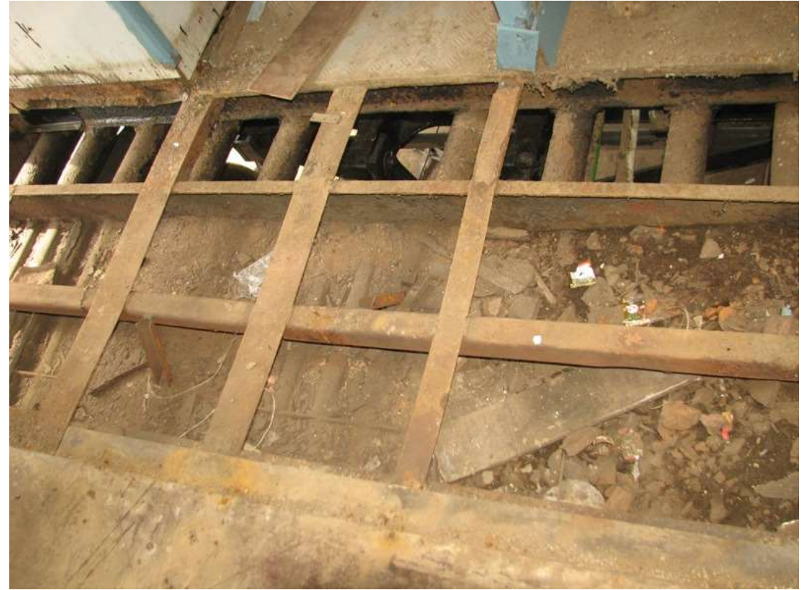
Corroded Door passage floor area
