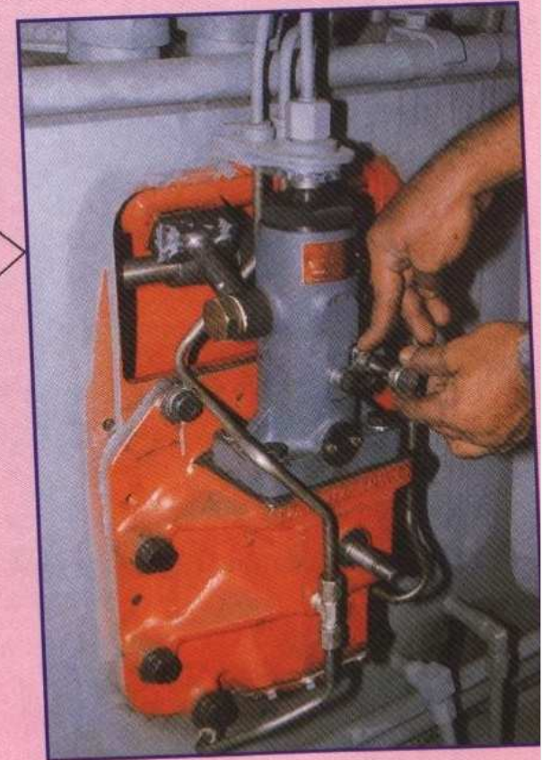
Photo.2 Lock Fuel Injection Pump Rack to stop the Leakage from High pressure pipe line.
